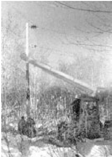
Utility crews worked for weeks after the 1978 blizzard repairing damaged equipment. Hingham utility employees use a timber jack to right downed poles.
